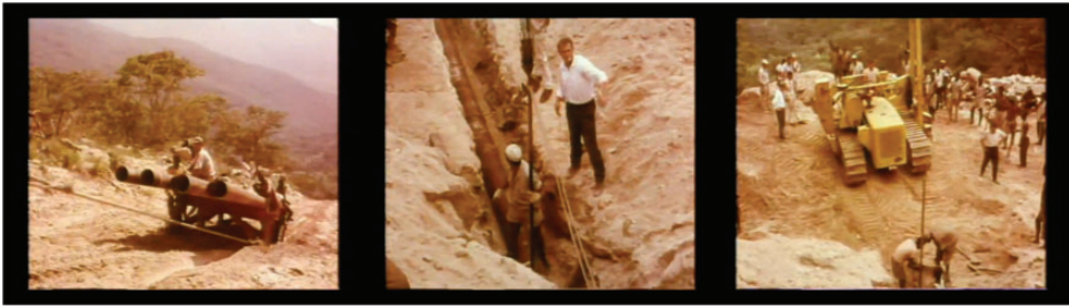
Figure 2. Scenes of the pipeline construction from “From the Indian Ocean to the heart of Africa: The oil pipeline Dar es Salaam–Ndola”, Raoul Brunlinger, 1969. Source: Eni Historical Archive.
