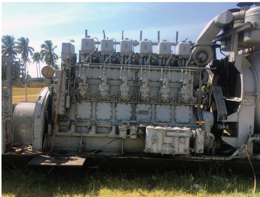
Figure 4. The pumping station of Iringa (Tanzania) after the bombing of 24 December 1968. As reported in The Standard Tanzania on 27 December 1969: “The explosion which ripped through the building blasted off the asbestos walls and roof leaving only a metal skeleton standing”. Source: F.L.i private collection.
